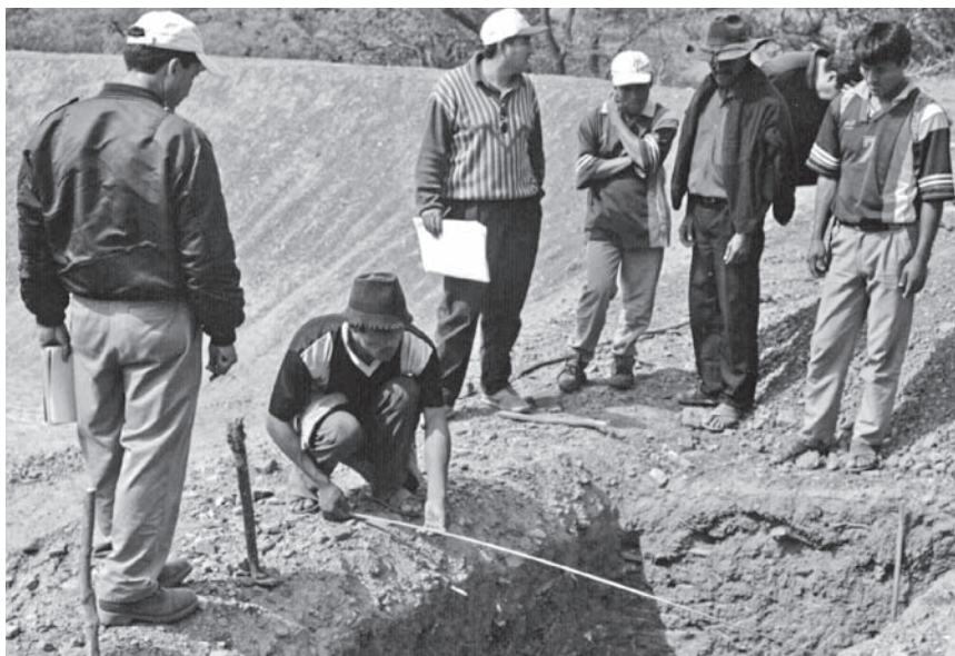
Farmers and service provider conduct quality control at water pond construction site.
