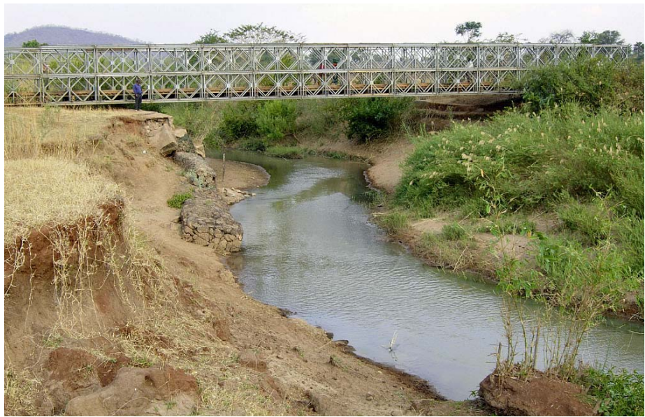
Endangered rural infrastructure: risks may be higher in the future (Songwe river, Tanzania). Photo: Udo Höggel
