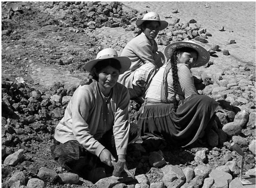
Participation of users in the construction of a new water system in Cochabamba, Bolivia.
